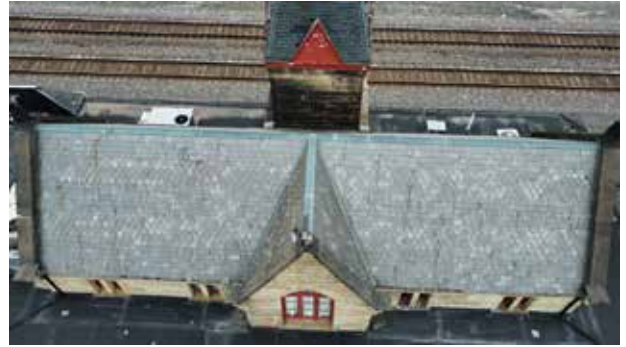
The backside of the tower is deeply stained from coal soot.
